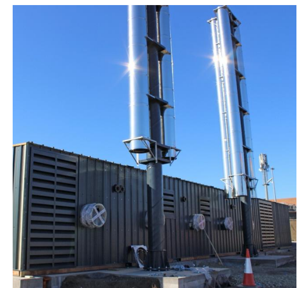
INTERIM ENERGY CENTRE
